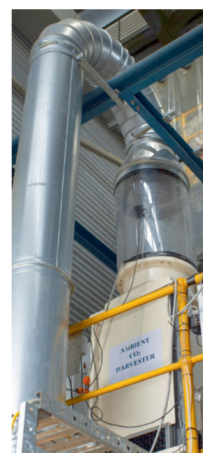
Figure 2: Ambient CO 2 Harvester (ACOHA) 4 tonnes CO 2 /annum demonstration located at the CSIRO Energy Center, NSW, Australia.
