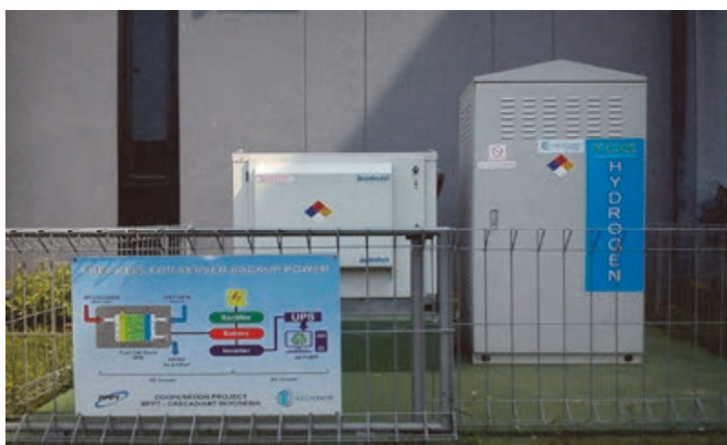
Fig. 1. PEMFC as BACKUP SERVER at Puspiptek
